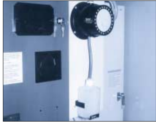
Hasselblad, the Swedish camera makers, have installed a number of OPUS silencers in their production to eliminate oil mist and impulse noise. This picture shows a CNC machine fitted with a CDO for oil separation.
