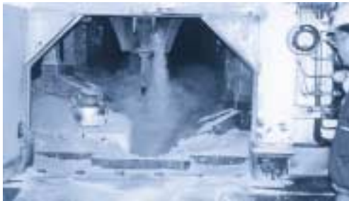
Hoogovens Aluminium Huttenwerk GmbH uses approximately 250 SILVENT 209 nozzles to cool the electrolyte in their furnaces. The company has 188 furnaces in operation.
