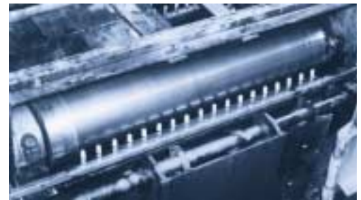
This picture shows a manifold with SILVENT 209 nozzles drying sheet metal at a steel mill in the USA. Previously, flattened open pipe was used to blow the steel dry. Installing SILVENT lowered the noise level by 50% and thanks to reduced air consumption, the installation paid for itself in less than 3 months.
