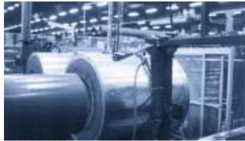
A compressed air cleaning station for plastic pipe. SILVENT 407 nozzles are mounted on a pneumatic rotor arm. The arm is automatically controlled and moves forward to the mouth of the long pipes prior to blowing clean. This installation resulted in both reduced air consumption and an improved working environment in the form of lower noise levels.
