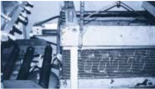
Here, a custom-made 300 manifold with SILVENT 209 nozzles is mounted in the final phase of the process in an industrial washing facility. The nozzles are intended to dry parts as well as to prevent methylene chloride fumes from spreading to the adjacent production area.
