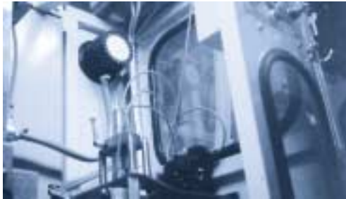
PLM's Plastic Division has implemented a noise control program in their production facilities. The company has installed more than 50 CDs in their blow molding machines and thereby effectively solved their noise problem and eliminated a previous problem they have had with clogged silencers.
